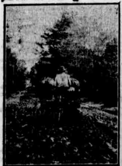
MIXING SAND AND GRAVEL. tries day. It is generally recognized by highway authorities and road users that the methods of building wagon roads with broken stone, as introduced by Telford and MacAdam a century ago, have become obsolete. While
